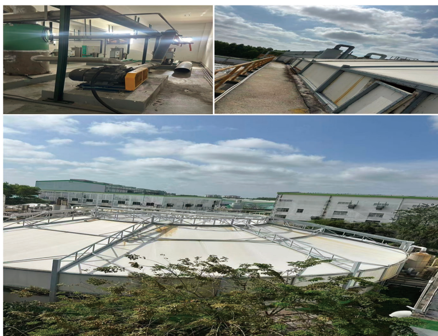
Ozone exhaust gas recycling system 臭氧尾氣回收系統
